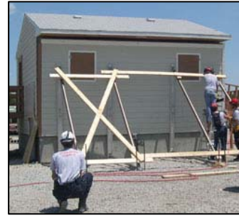
Structural Collapse Rescue Training
