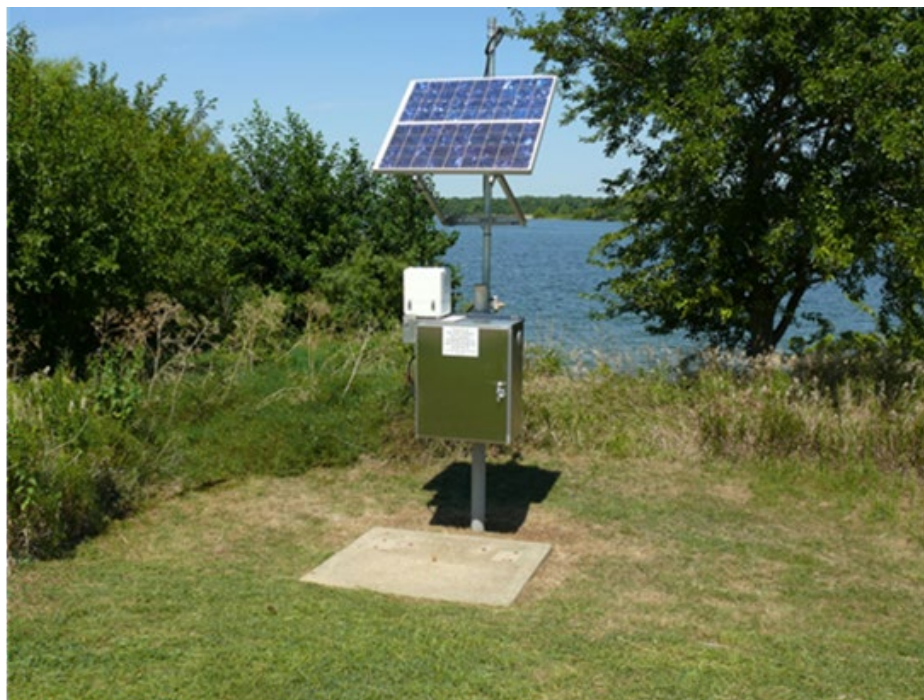
Figure 6. Typical IEMA GDN Field Installation
