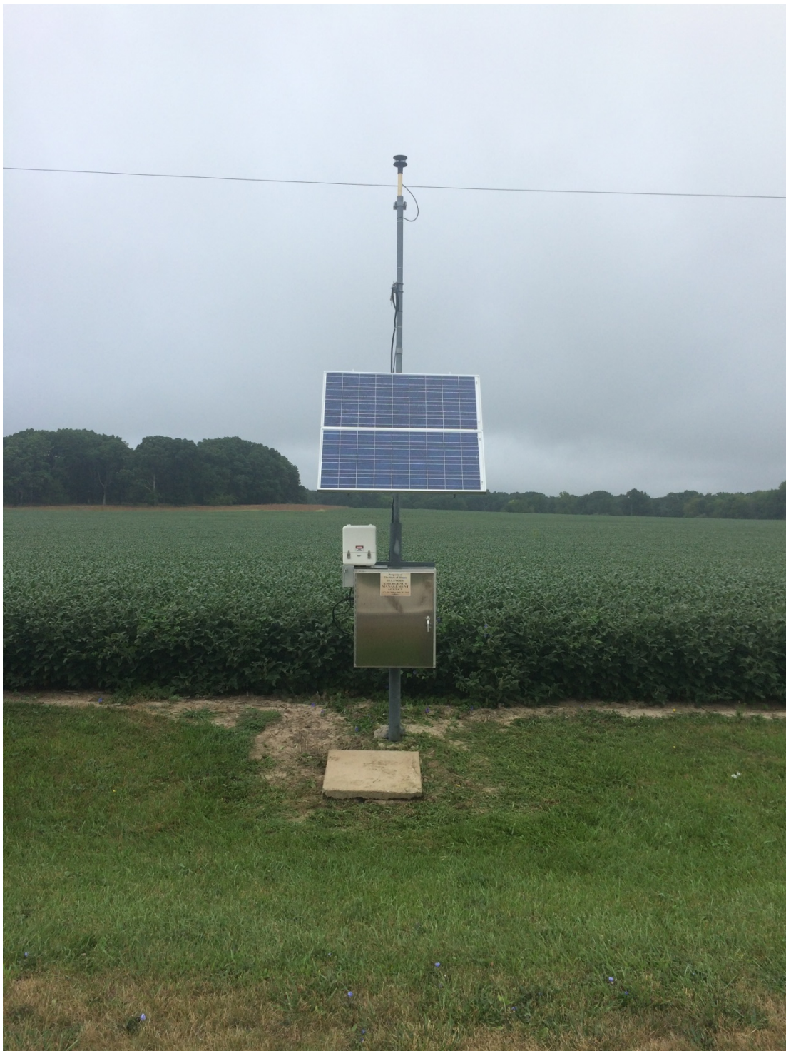
Typical IEMA GDN Field Installation
